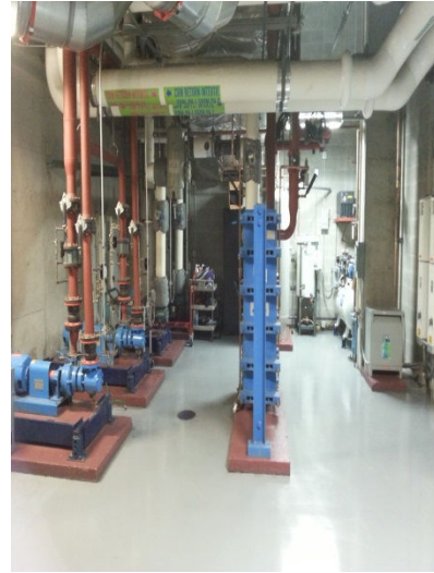
The heated water return
