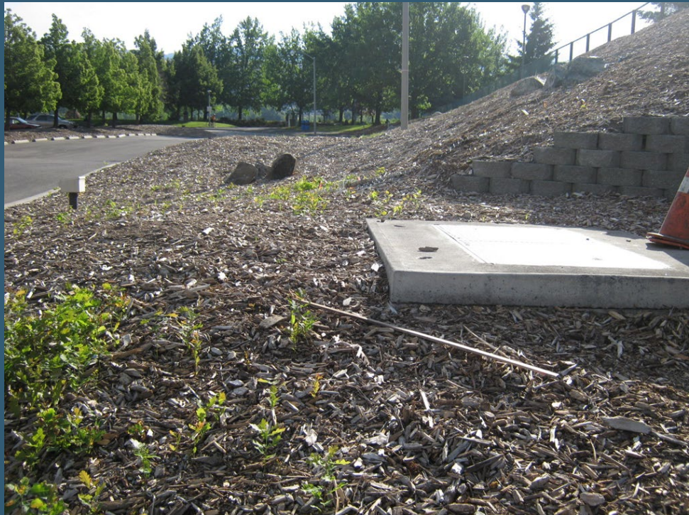
DCVA Vault at PUD Parking Lot on Worthen Street
